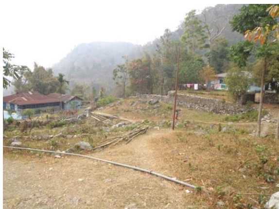
Plate 2: Pipe line drinking water facility at Chunabati village
