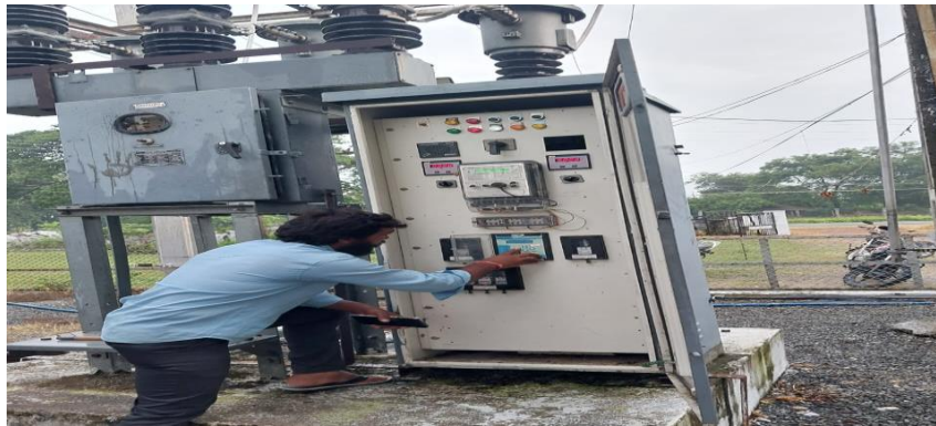
Figure 1: Feeder readings recording in the feeder circuits by a lineman in a substation
