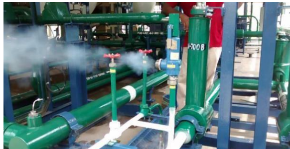
Fig. 2.1 Cryogenic PRV in operation at LSSF
