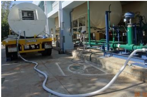
Fig.4.2 Liquid nitrogen storage tank at operation
